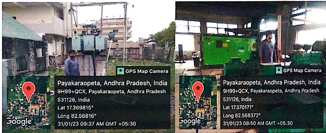
Electrical power station
